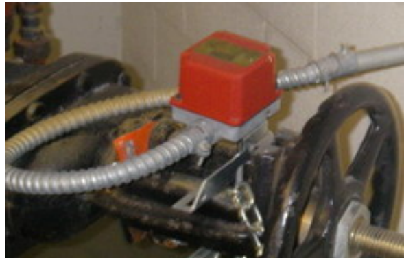
Tamper switch on a sprinkler valve
